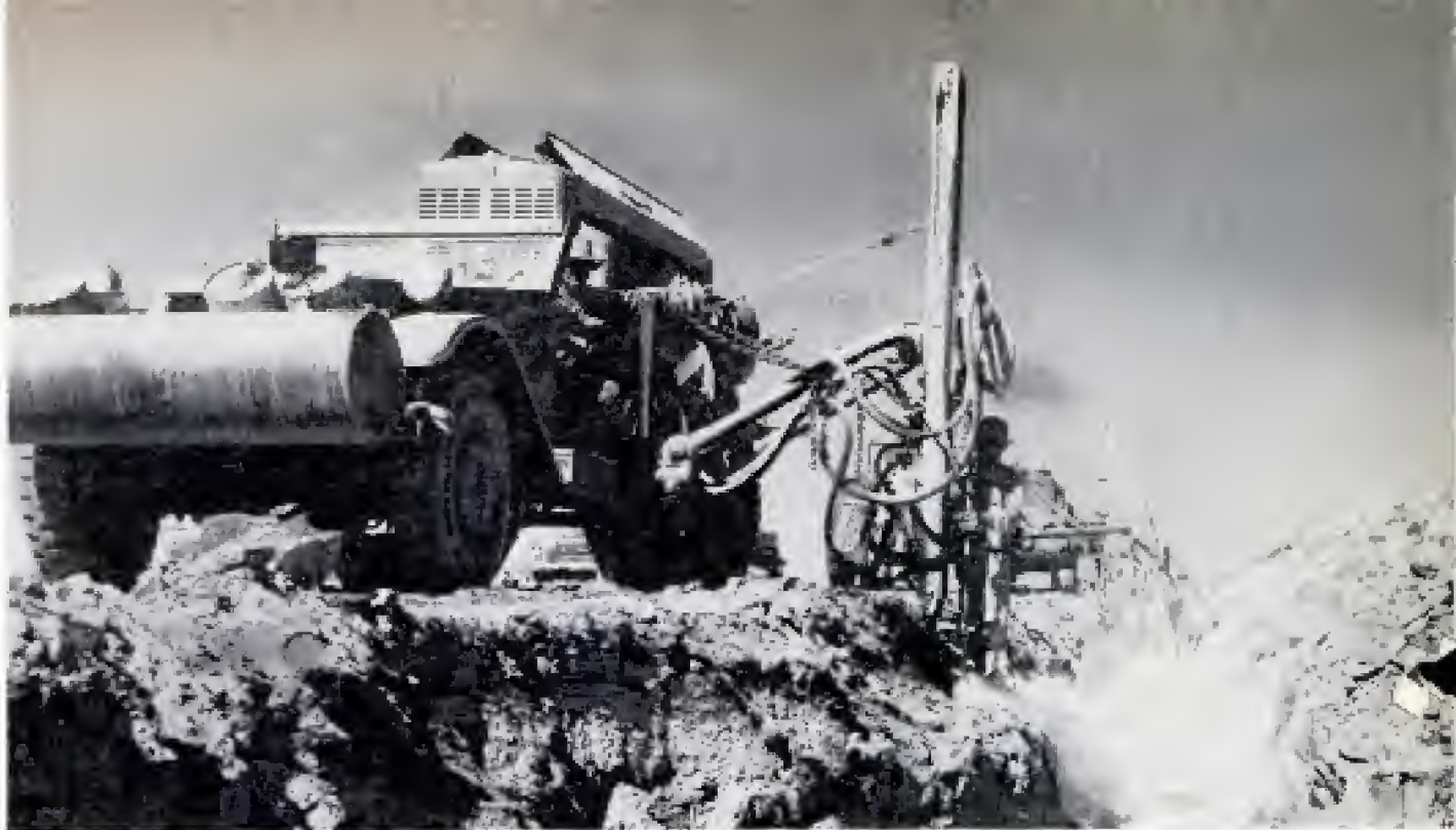
At the archeologists' beck and call were units like this Army truck fitted with compressors and drills
